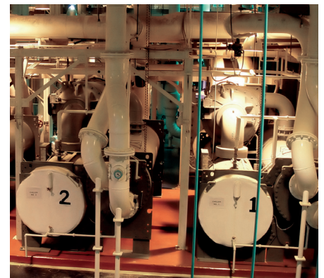
Figure 3. Two 15-Ton Chillers
